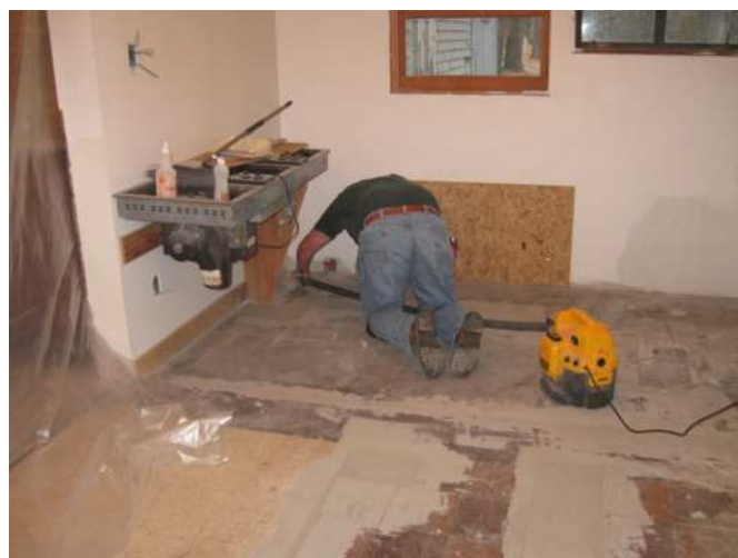
The previous kitchen floor was conglomeration of different surfaces, cement, tile, missing tiles and wood. In this photograph, Ken is vacuuming up some of the debris after leveling the floor.
