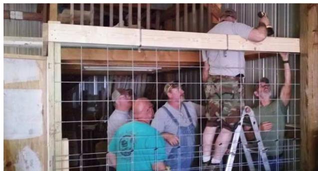
Frank, Dave, Ken Vince and Jim discuss putting a ceiling on the nearly completed storage area.
