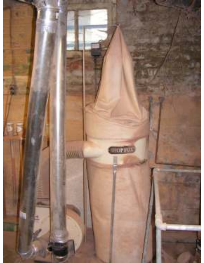
Dust collection systems take up a lot of space in a shop and have ducts connected to each dust producing tool.
